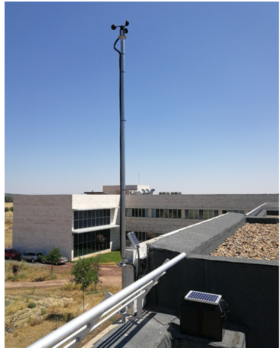
Fig. 3. Testbed installation at University of Castilla-La Mancha in Ciudad Real, Spain (38°59'00"N, 03°56'00"W).
